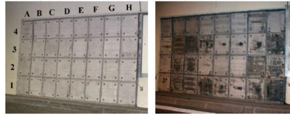
Fig. 4: Visual state of the concrete test panels in the Naxberg tunnel in the year 2000 (left) and 2012 (right).
